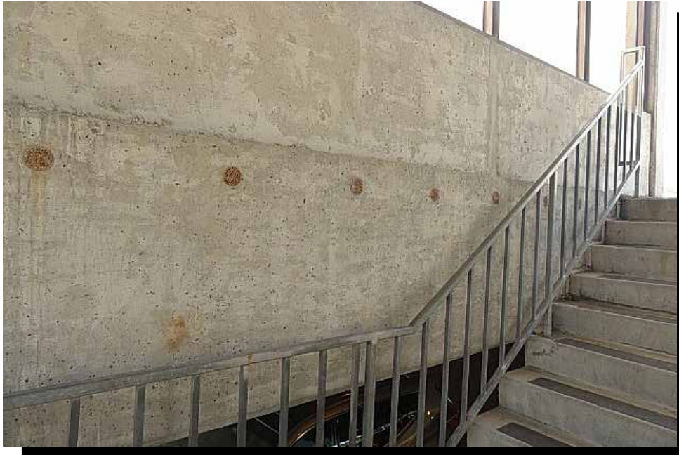
Figure 4: Corrosion at Slab Grout Pockets
