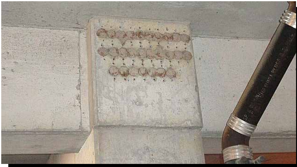
Figure 5: Corrosion at Beam End Grout Pockets
