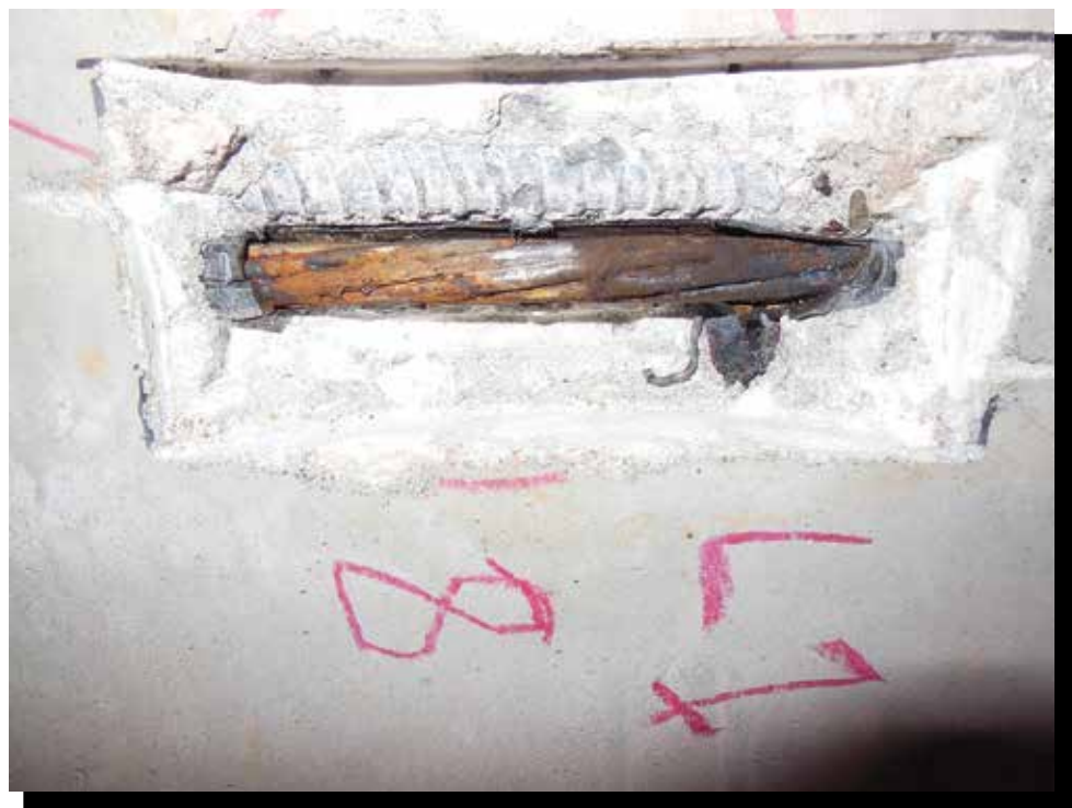
Figure 3: Severe Corrosion and Degraded Grease
