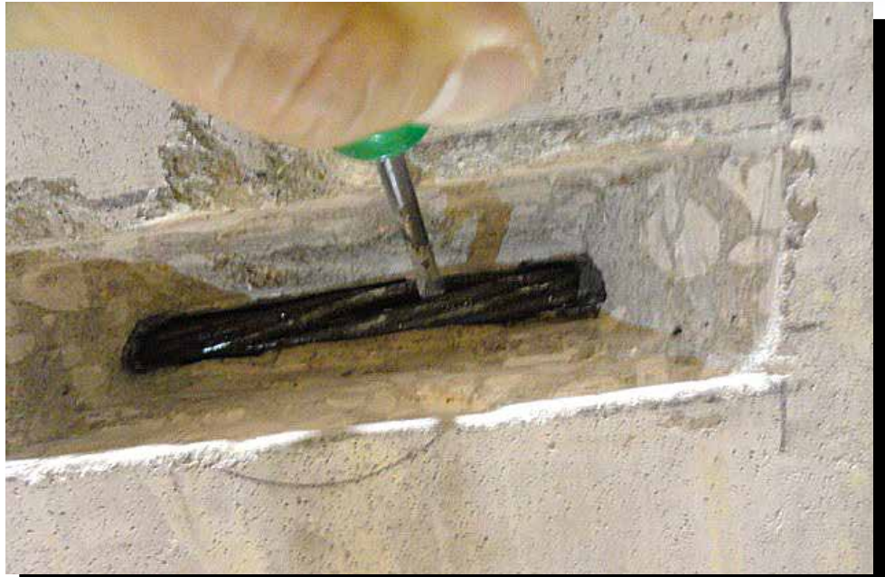
Figure 2: Screwdriver Penetration Test Detecting Broken Wires
