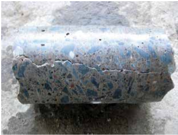
Core Sample Showing Full-depth Cracking
