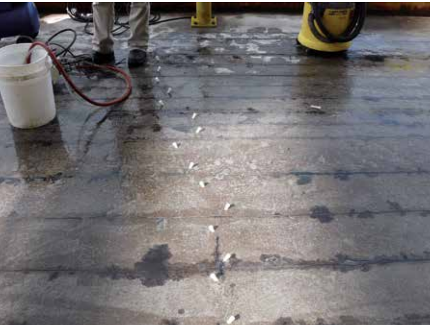
Ports Installed for Cleaning / Injection
