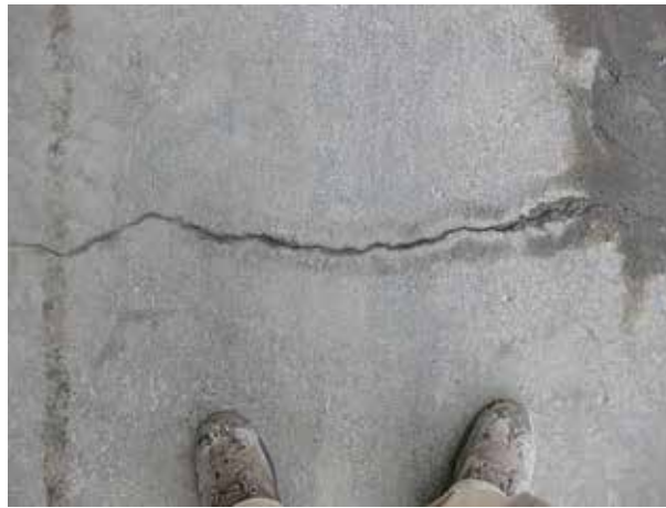
Typical Negative Moment Crack Over Beams
