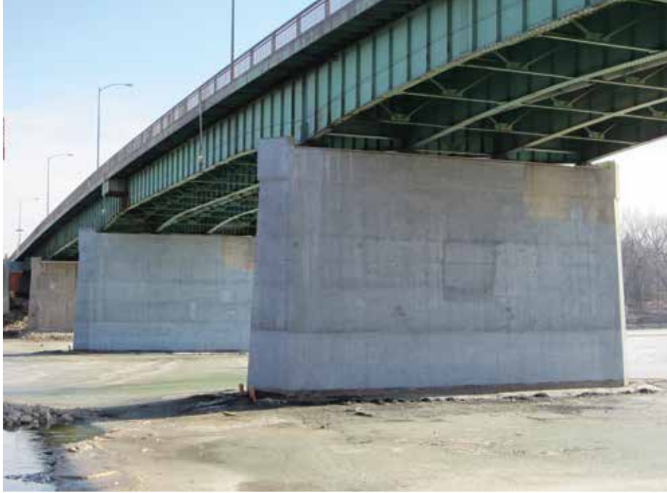
Humectant Activated Arc Sprayed Zinc was used to Protect the Two Interior Piers
