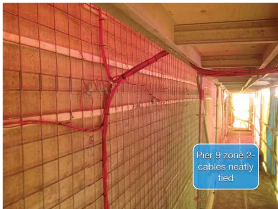
Temporary Anode Mesh and Wiring in Place for Electrochemical Chloride Extraction Treatment for the Two Land-Based Piers
