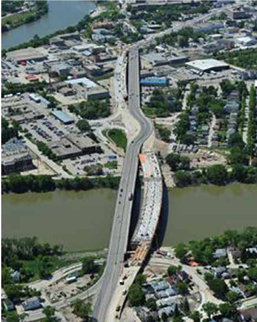
Aerial View of the Disraeli Bridges Project over the Red River with Traffic Diverted onto the New Bridge
