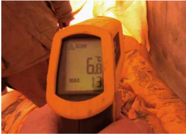
The Heated Enclosure Allowed Work to Proceed Despite Exterior Temperatures as Low as -30°C
