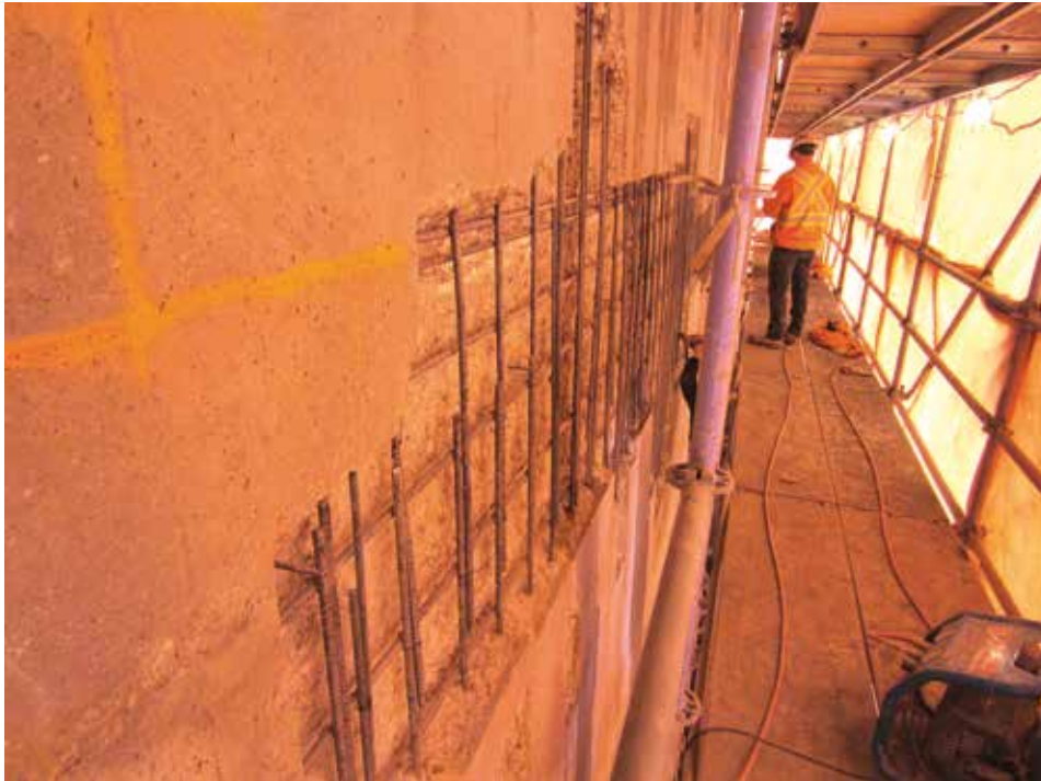
Example of Corrosion Damage on Red River Bridge Piers
