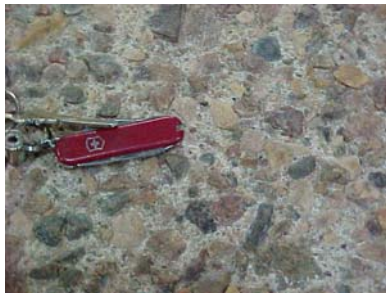
Existing Concrete Condition
