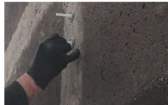
After the surface has been cleaned, surface-mounted injection ports are installed. A temporary crack-sealer epoxy paste will be applied on the face of the crack between and around the ports before the injection process begins.
